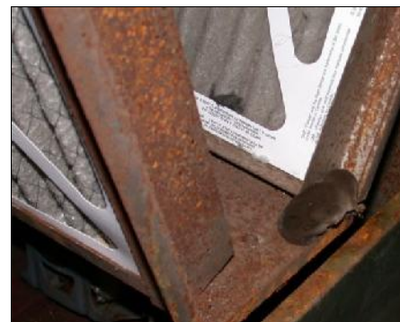
Dead shrew in air handler May Indoor Air Investigations LLC
