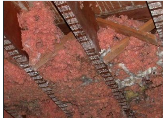
Circular mouse burrows in garage insulation May Indoor Air Investigations LLC
