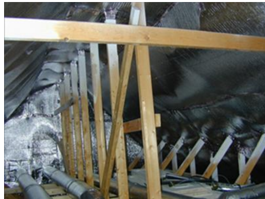
SPF in attic, covered with foil to prevent off-gassing May Indoor Air Investigations LLC
