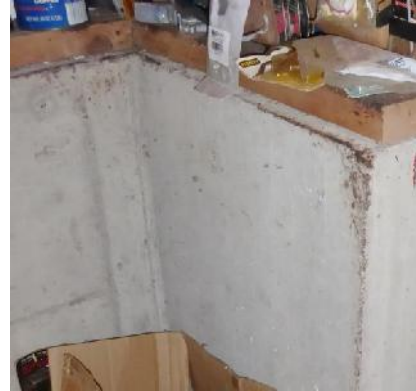
Rust-colored mouse-urine stains on concrete edges May Indoor Air Investigations LLC
