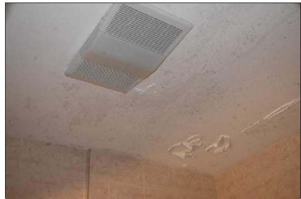
Bathroom ceiling with peeling paint and spots of mold growth
