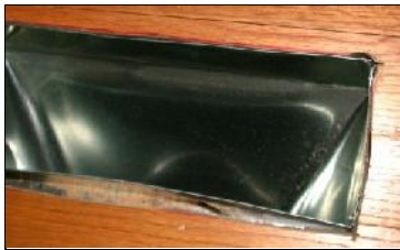
Gap around boot in duct leading from crawl space May Indoor Air Investigations LLC
