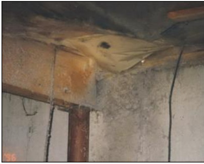
Severe mold growth around a dryer vent exhausting into a crawl space May Indoor Air Investigations LLC
