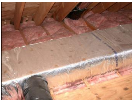
Drip stains on attic duct and fiberglass from house moisture condensed on roofing nails May Indoor Air Investigations LLC
