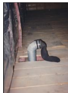
Dryer "sock" in attic May Indoor Air Investigations LLC
