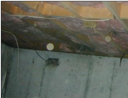
Moldy joists and fiberglass in crawl space May Indoor Air Investigations LLC
