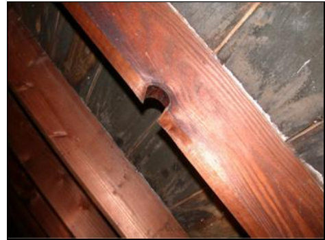
Mold growth on attic sheathing May Indoor Air Investigations LLC
