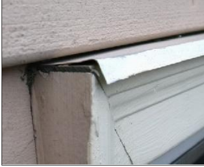
Cap flashing with improper pitch and open joint May Indoor Air Investigations LLC
