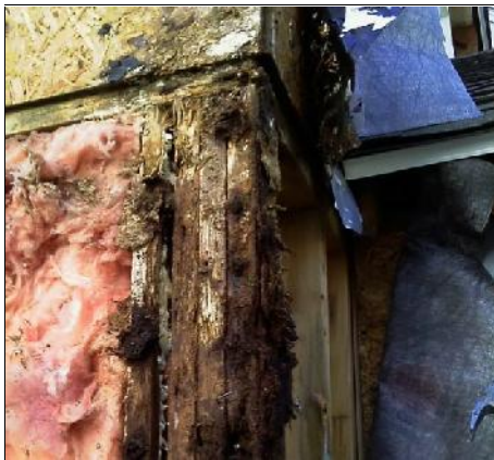
Decayed sheathing and corner post May Indoor Air Investigations LLC
