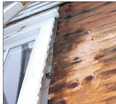
Decayed sheathing behind clapboards May Indoor Air Investigations LLC
