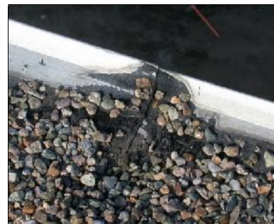
Gap in roof flashing May Indoor Air Investigations LLC
