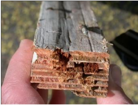
Decayed vertical casing after removal May Indoor Air Investigations LLC
