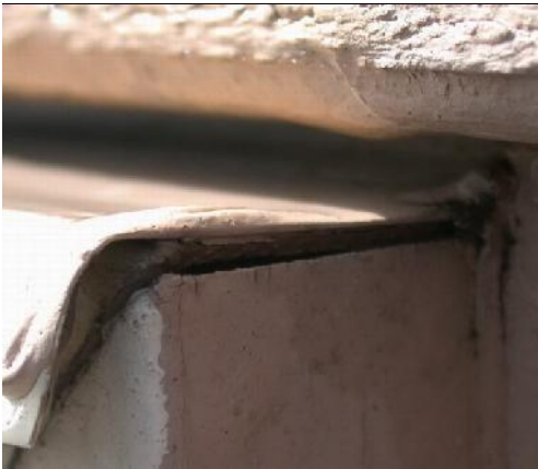
Test water entering miter joint May Indoor Air Investigations LLC
