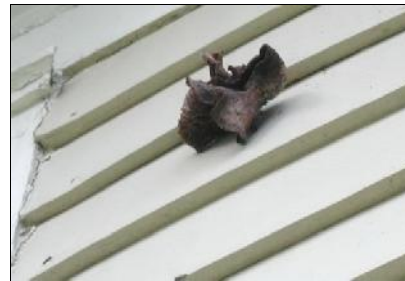
Mushroom on hardboard siding May Indoor Air Investigations LLC
