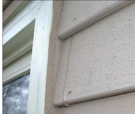
Test water exiting clapboard May Indoor Air Investigations LLC
