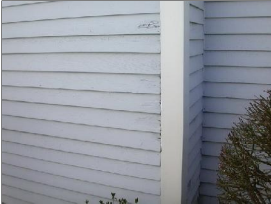
Visible siding decay at exterior corner May Indoor Air Investigations LLC
