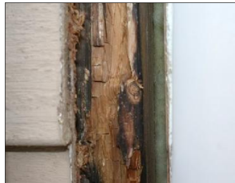
Stud decay at behind casing May Indoor Air Investigations LLC
