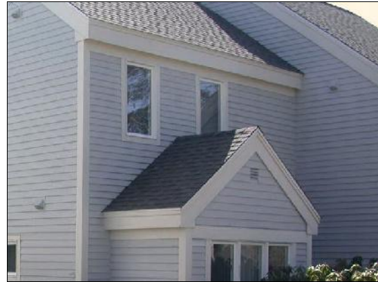
Large volume of roof water flows from upper gable onto lower gables May Indoor Air Investigations LLC
