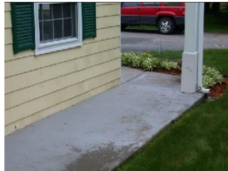
Woops! What's wrong with this picture? Gutter-system maintenance is important!
