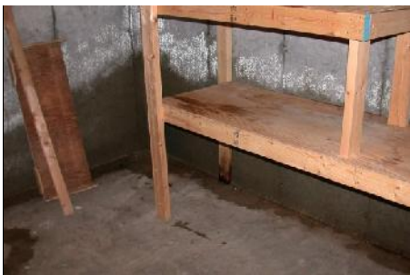
Moisture stains and efflorescence point to basement water intrusion
