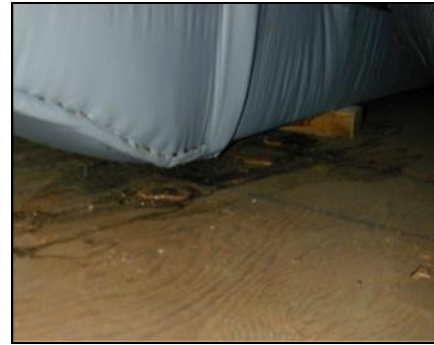
Leak stains under duct from condensation within
