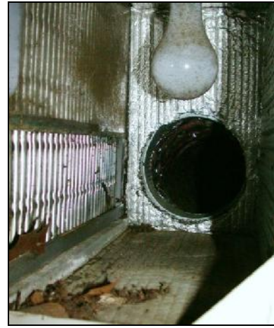
Mold growth on the intake side of an old-style HRV
