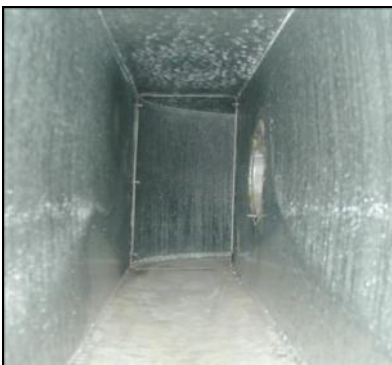
Condensation in attic A/C supply duct
