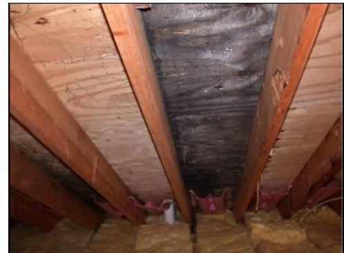
Mold growth due to air back-drafting into attic soffit
