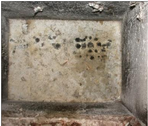
Visible mold growth in return plenum due to leaking humidifier May Indoor Air Investigations LLC
