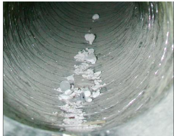
Construction debris in duct in newly built home May Indoor Air Investigations LLC
