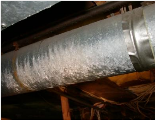
Condensation on metal duct May Indoor Air Investigations LLC
