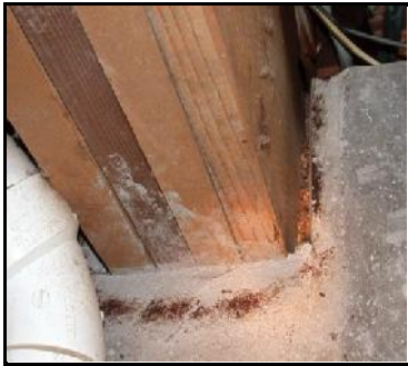
A mouse-urine trail around a beam May Indoor Air Investigations, LLC
