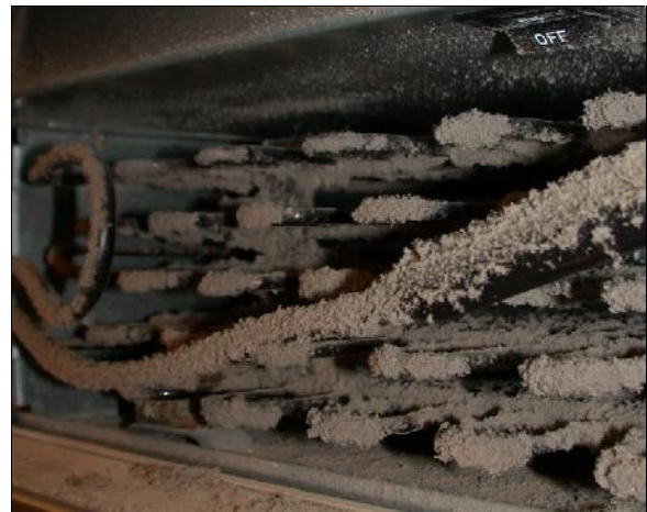
Dirty refrigerator coils May Indoor Air Investigations LLC
