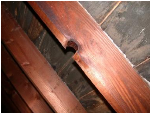
Attic sheathing with mold growth May Indoor Air Investigations LLC
