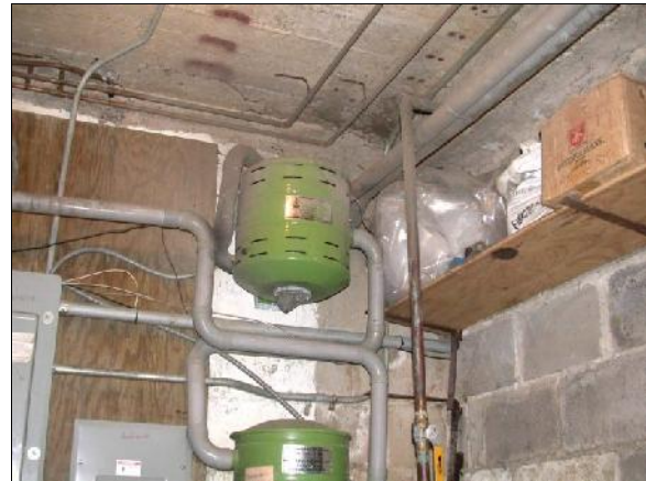
Leaky central vacuum system May Indoor Air Investigations LLC
