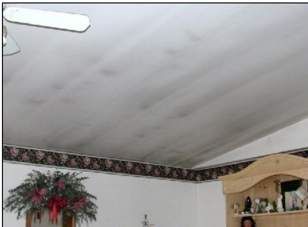
Candle-soot stains on a ceiling denoting insulation gaps
