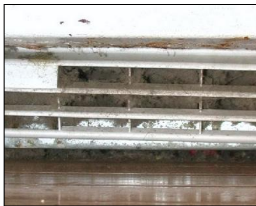
Potentially allergenic dust on refrigerator coils
