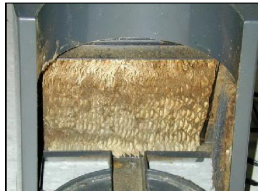
Pad in evaporative humidifier, with cigarette tar and Aspergillus mold
